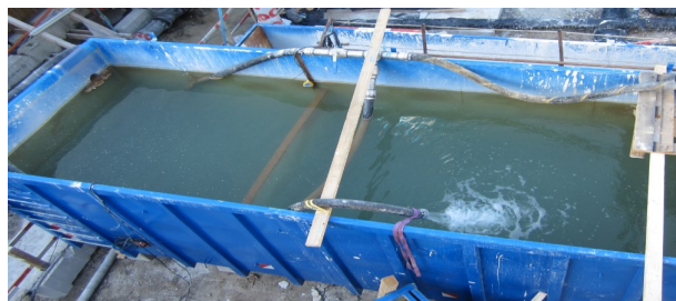
Picture 2: Ground water from construction site in settling tank (prior to UF membrane treatment)
