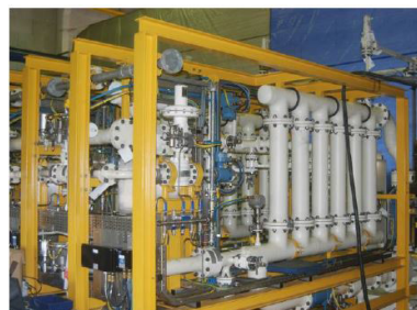
Case 1 - Final installation with LiqTech's SiC membranes
